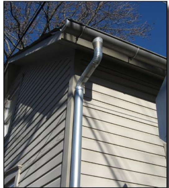
Half-round gutters and downspouts are recommended for Clarksville’s historic dwellings (424 S. First Street).
